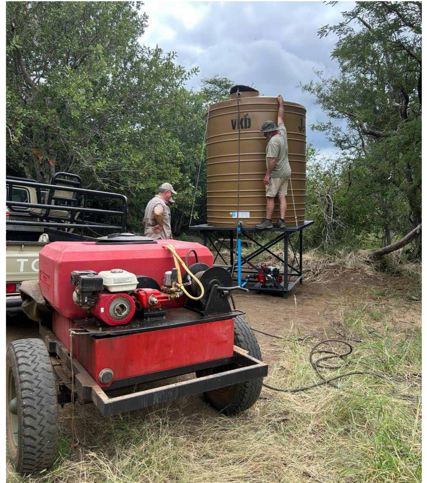
A 500 litre mobile tanker to supply water to the installed tank and also provide firefighting ability
